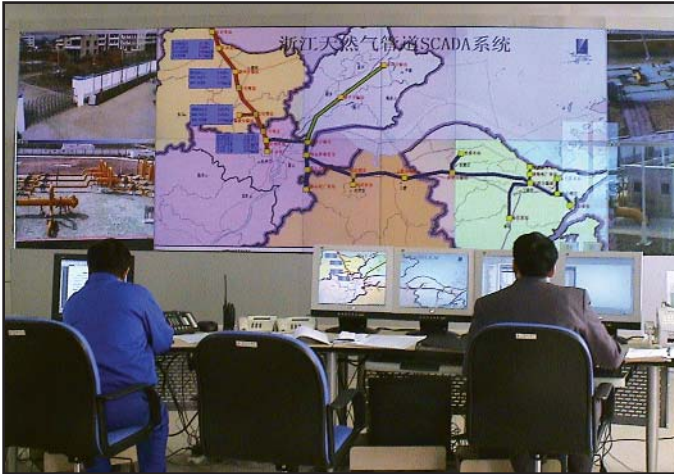
Control room at Zhejiang Natural Gas Co.
